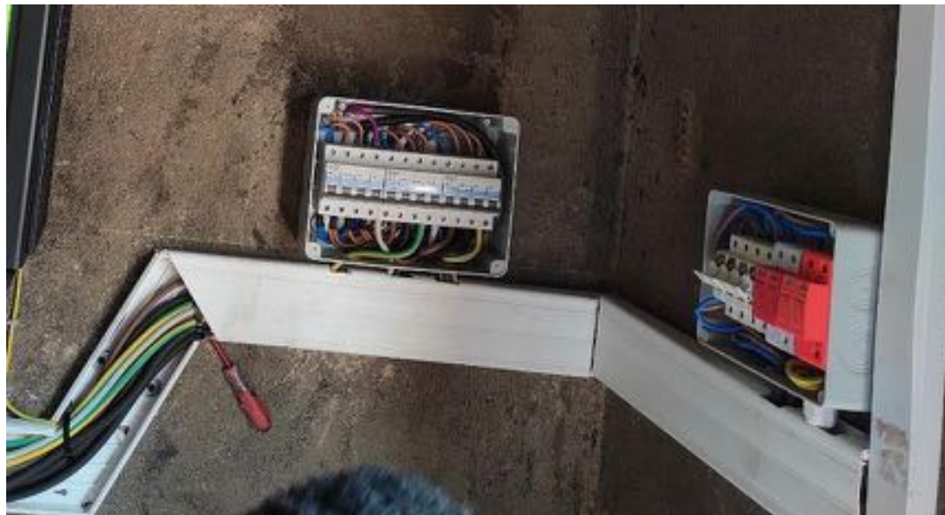
Figure 19 : System protection equipment
