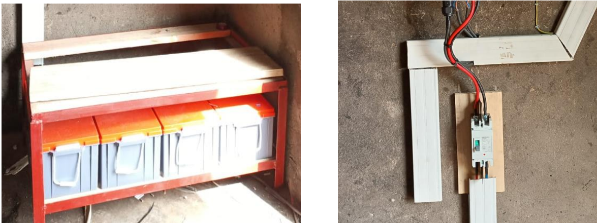
Figure 7 : Batteries plus protection
